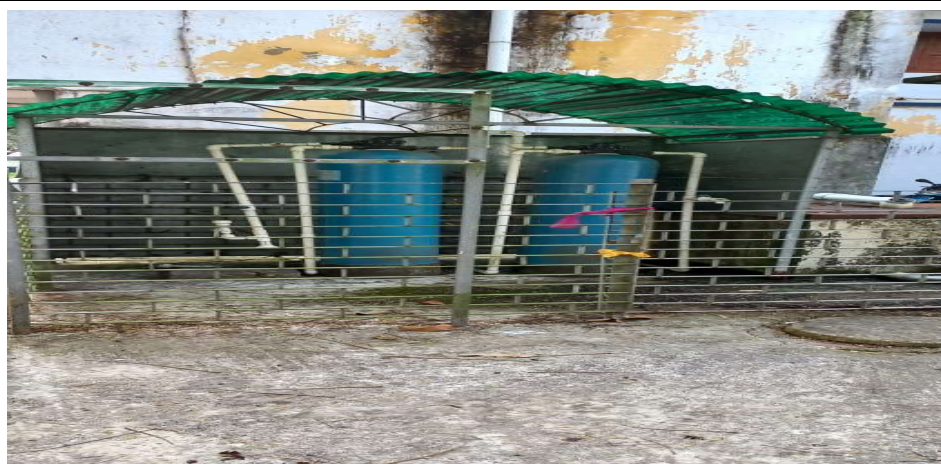
Rain water harvesting System Installed
